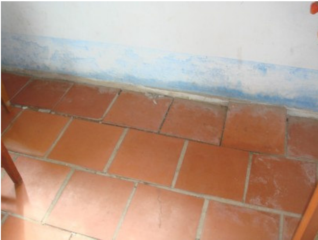
The foundation in the current building is sinking.
